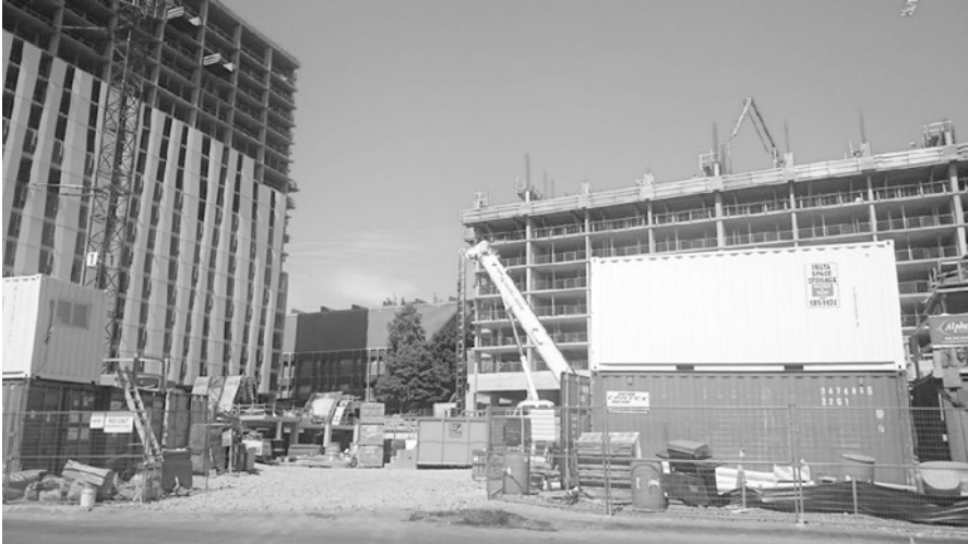
Fig. 8.3 Destruction/construction site of the original UBC Orchard Garden/new Orchard Commons. (Photo credit: Sandra Scott)
