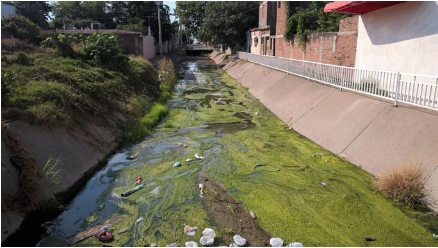
Fig. 21.2 The urban drainage ditch is carrying several types of waste ( picture Otoniel Carranza)
