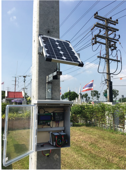
Fig. 7. The LoRa base station
