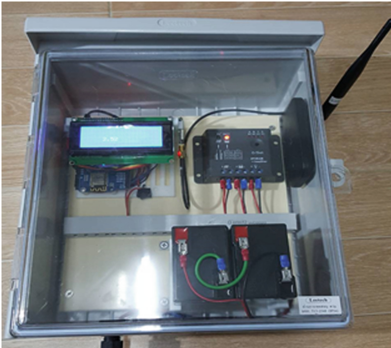
Fig. 10. The master node with solar panel on high-voltage
