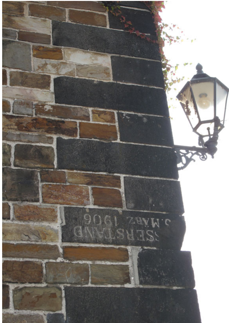
Fig. 10.16 Reused stone with turned over flood level mark at the foundation of a railway bridge in Koblenz/River Rhine. Photograph Herget
