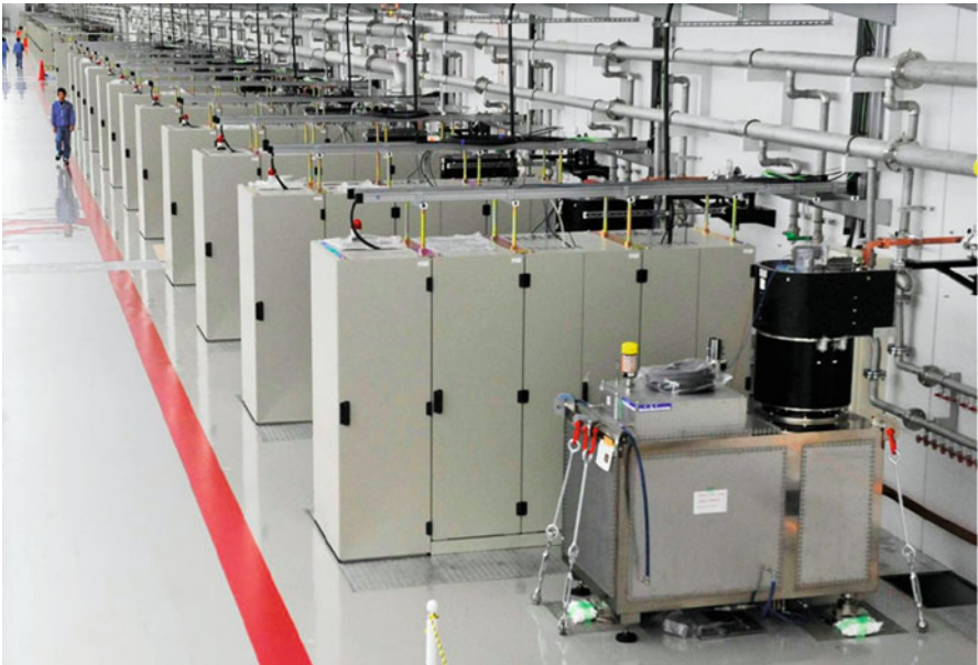
Fig. 3 Klystron gallery houses 72 C-band klystrons modulators and associated controls, 8 S-band klystrons and modulators, and power supply for the electron injector
