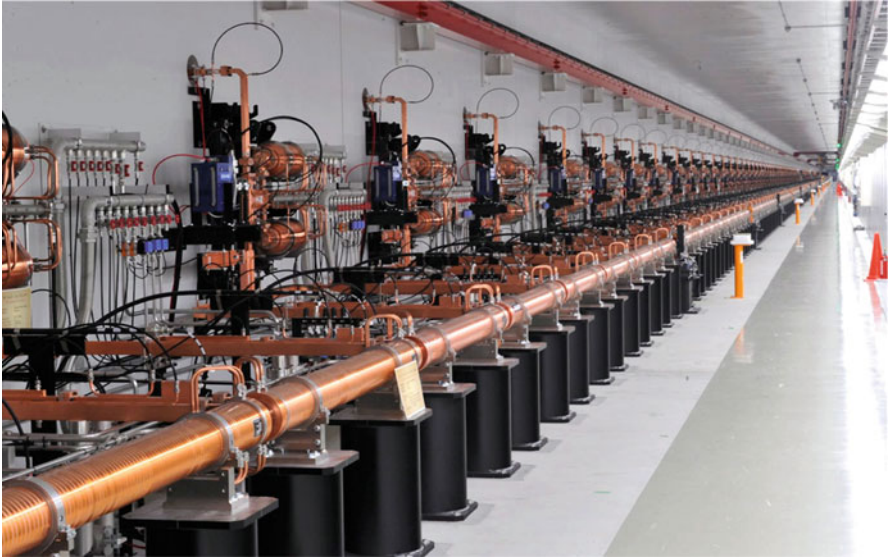
Fig. 2 C-band high-gradient accelerator in 400-m tunnel. A total of 128 accelerating structures have been installed to accelerate beams up to 8 GeV. Eight S-band accelerating structures are used in the injector part
