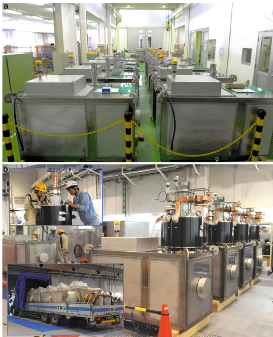
Fig. 27 (a) Mass production of the modulator in a factory. (b) Transportation and installation of klystron at SACLA site
