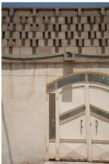
c. Lattice parapet in labourers' houses providing night time habitable space at roof
