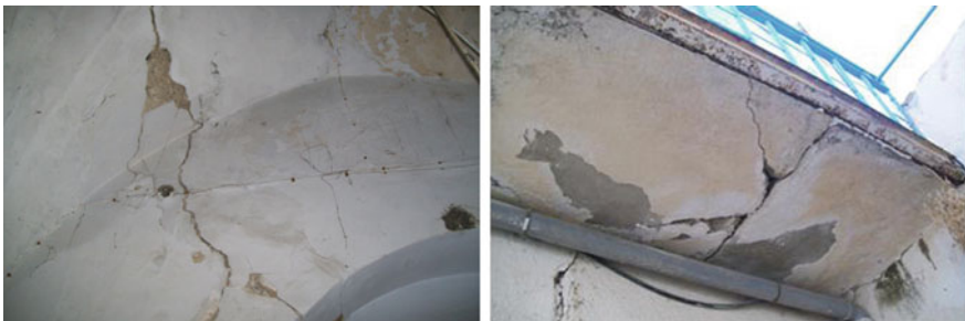
Fig. 10.3 The cracks that appeared after war. Source Authors
