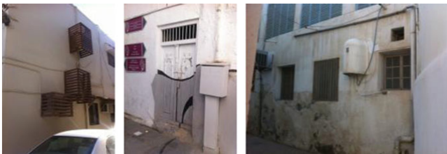
Fig. 4.14 Missing of using LA to cover the engineering facilities
