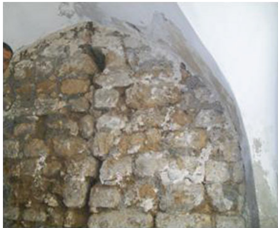
Fig. 10.12 A visible crack
