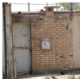
e. Built-in rubbish disposal boxes in labourers' quarters
