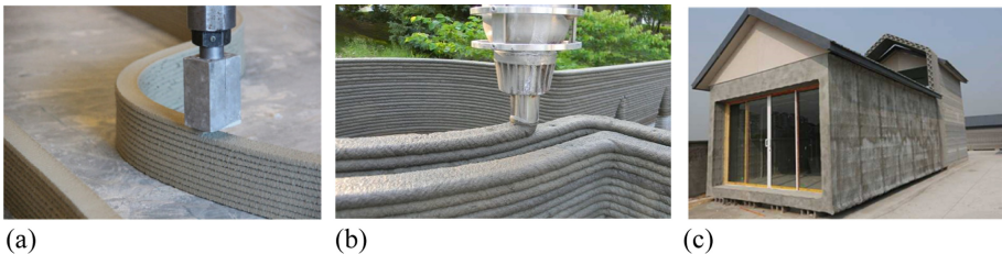
Fig. 4. 3D printing by layered extrusion: (a) Eindhoven University of Technology and (b) Andrey Kudenko, a contractor; and (c) Yingchuang Building Technique (Shanghai) Co., Ltd. (Winsun).
