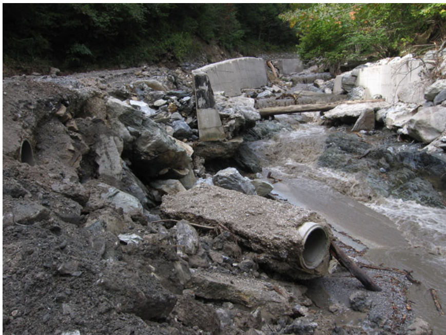
Fig. 3.17 Impact of a torrential flood in the Davča Valley in 2007 Photo Matija Zorn
