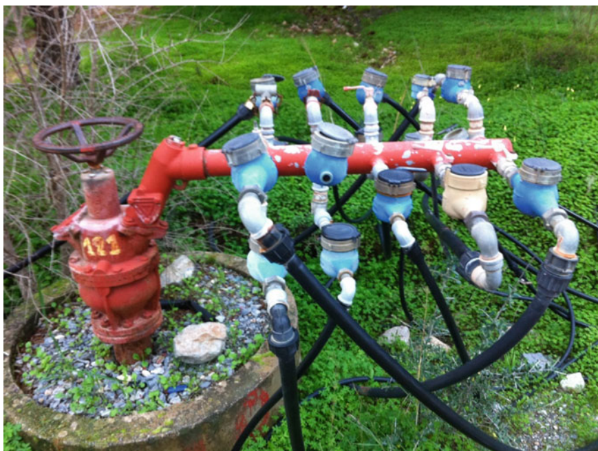
Fig. 16.9 Hydrant with 12 outlets in Crete. (Stefopoulou 2013)
