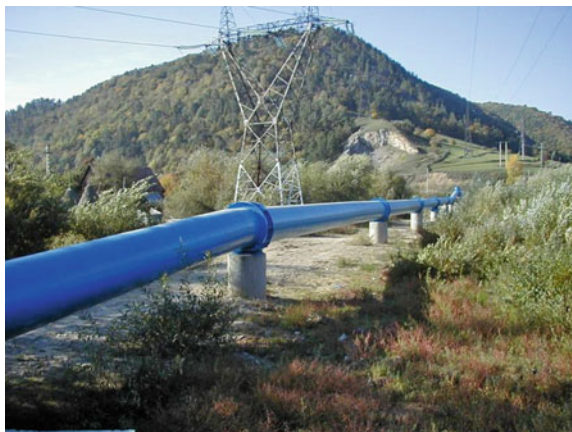
Fig. 6.1 The raw water supply pipe between Someșul Cald Lake and the Gilău WTP (photo by courtesy of CAS S.A.)
