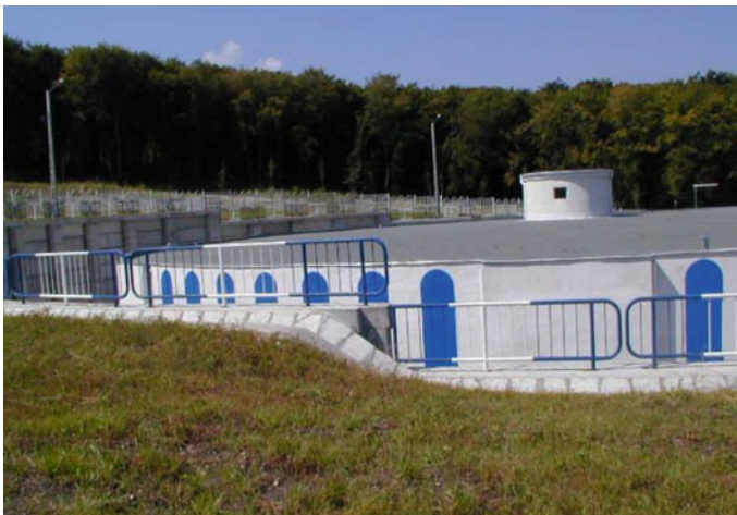
Fig. 6.3 A water tank built during MUDP II program (photo by courtesy of CAS S.A.)
