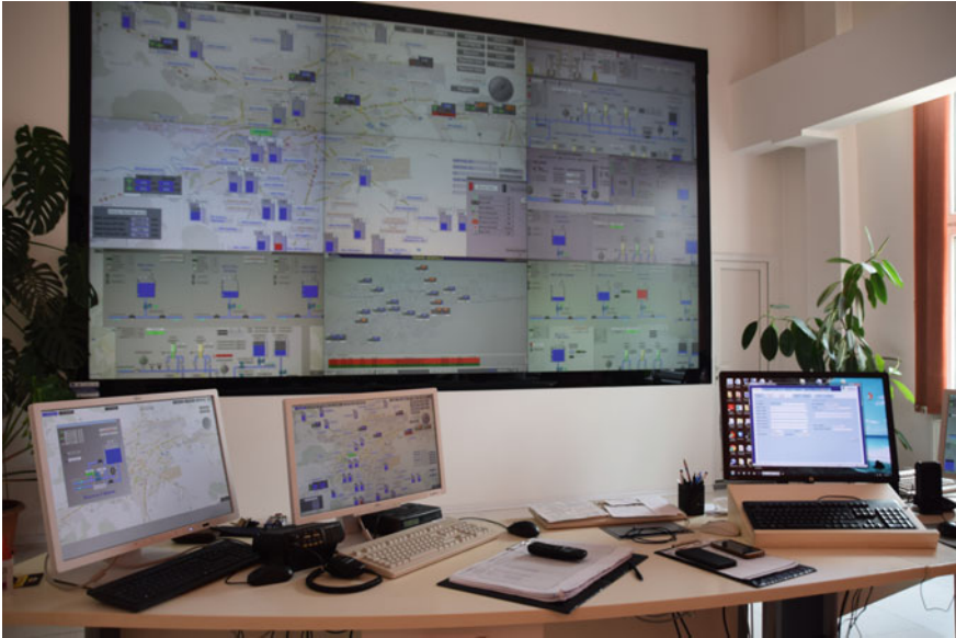
Fig. 6.10 SCADA in the Cluj-Napoca central dispatcher (photo by courtesy of CAS S.A.)
