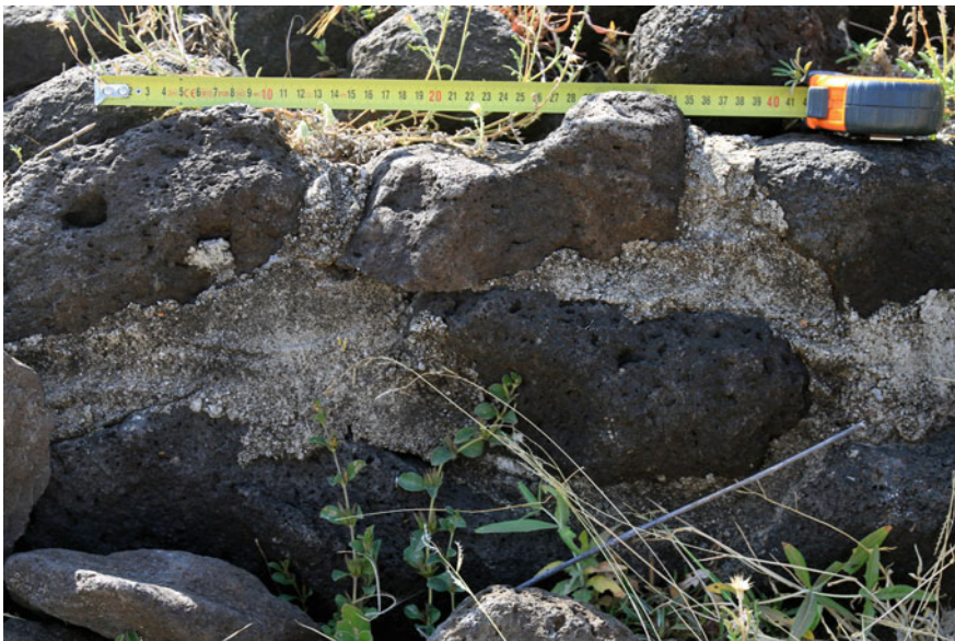
Fig. 36.5 Dark-coloured biofilms on the surface of concrete. Footprint conservation mound
