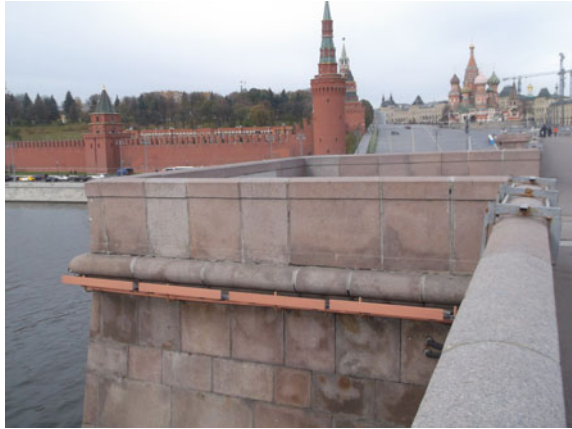
Fig. 28.4 Moskvoretskiy most. General view of the bridge abutment, visible rust stains, salts, crystal crusts
