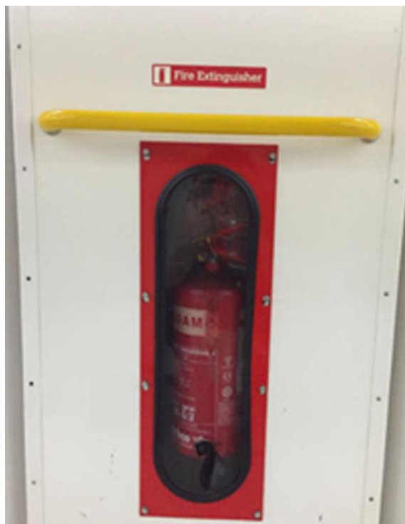
Fig. 6 Fire extinguisher casing on-board metro
