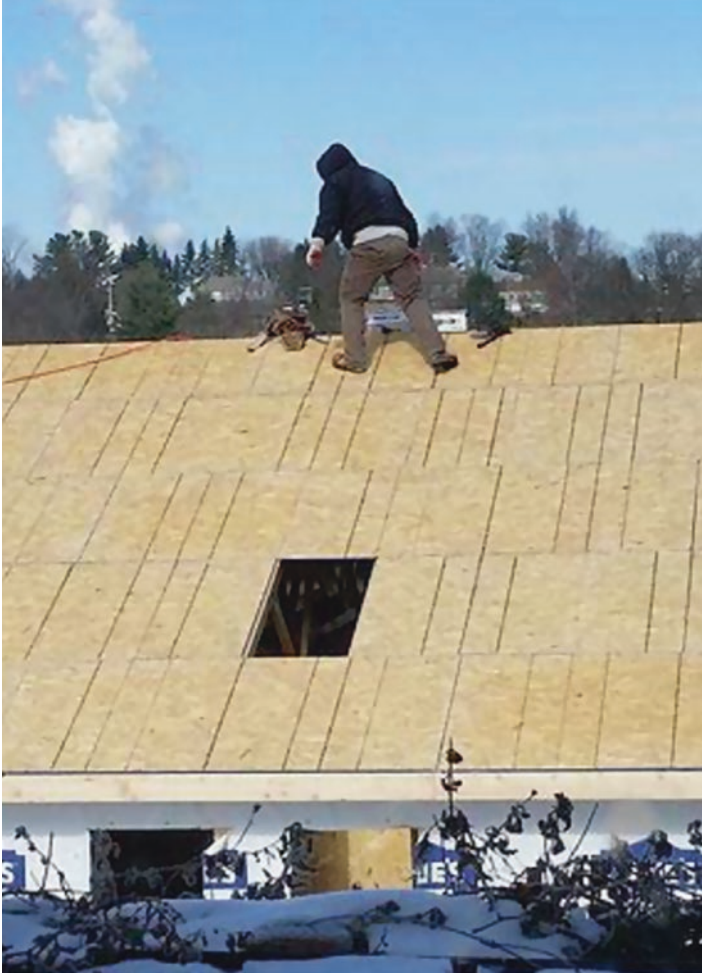
Fig. 8.1 Worker with no fall protection and clear hazard of falling from this roof. (Image: Winn 2016)
