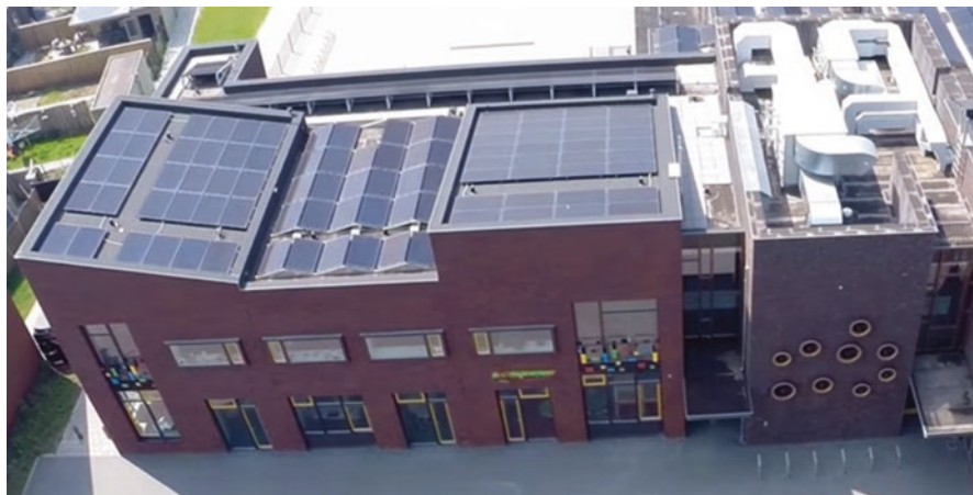
Fig. 15.4 Overview energy generation by PV panels of school 1 [9]
