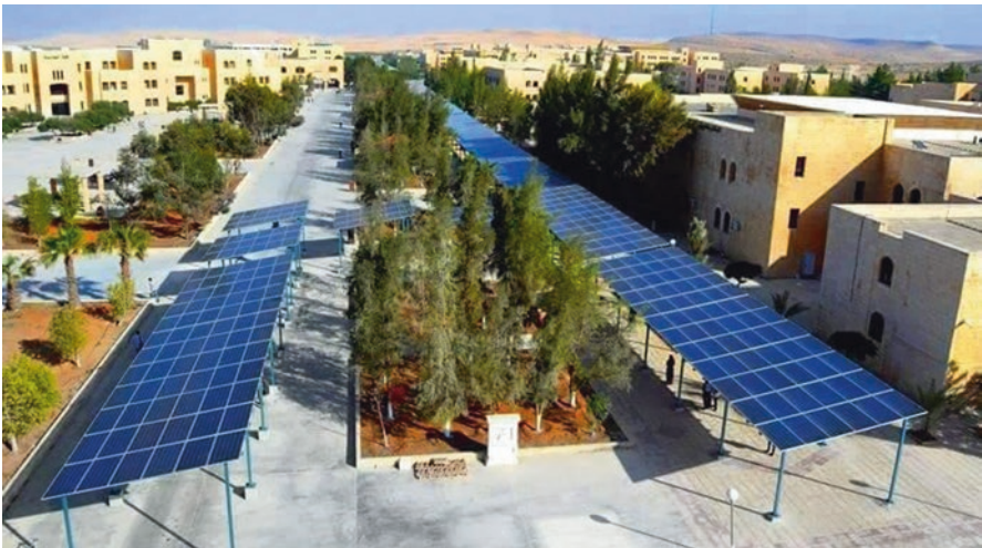
Fig. 52.3 A good example of the photovoltaic panels placed on the roof of a passage at the Hashemite University. It was highly accepted by people (source: albosala.com )
