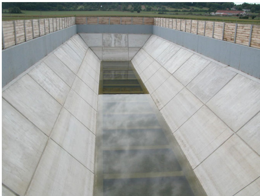
Fig. 7.11 Artificial infiltration in Ivančice spring area
