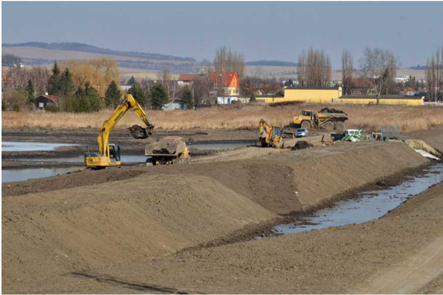
Fig. 15.7 Building of flood protection wetland near Slavkov u Brna. (Photograph: Jiří Schneider)
