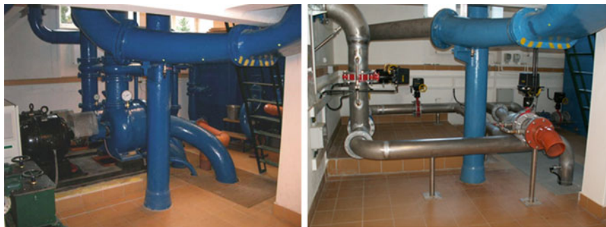
Fig. 2.15 Original pumping station (left) and pumping station innovated in 2008 (right)
