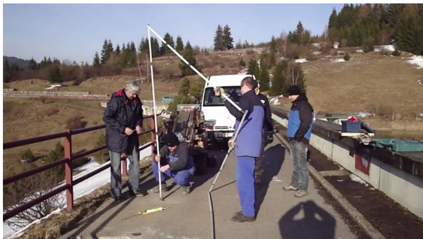
Fig. 2.24 Installation of EIS probes into the earth-fill dam of the Karolinka water reservoir jointly with the representatives of the company GEOTest, a.s
