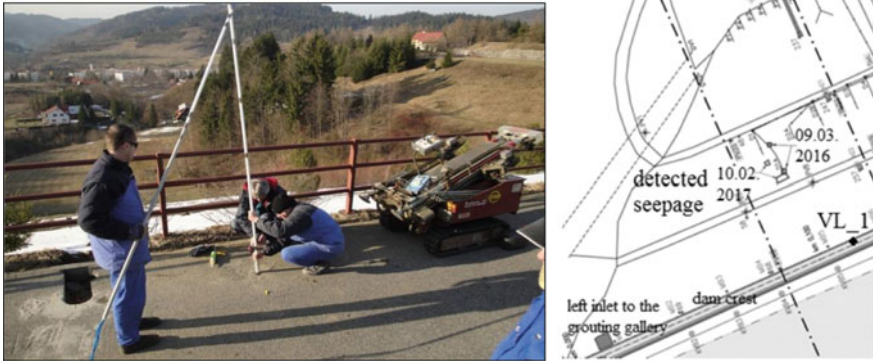
Fig. 13.7 Installation of probe VL_4 of the EIS method into the dam's sealing core (left), detected seepage sites after 2013—an outline of the situation (right)
