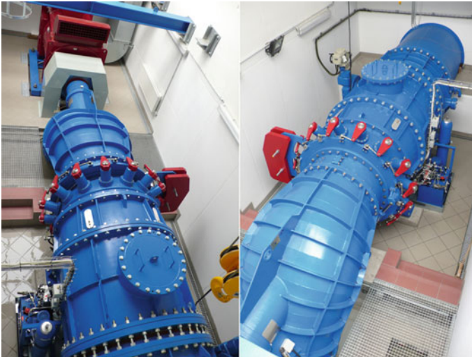
Fig. 15.23 Horizontal axial S-type Kaplan turbine in the SHPP Rozkoš (source Hydrohrom, s.r.o.)
