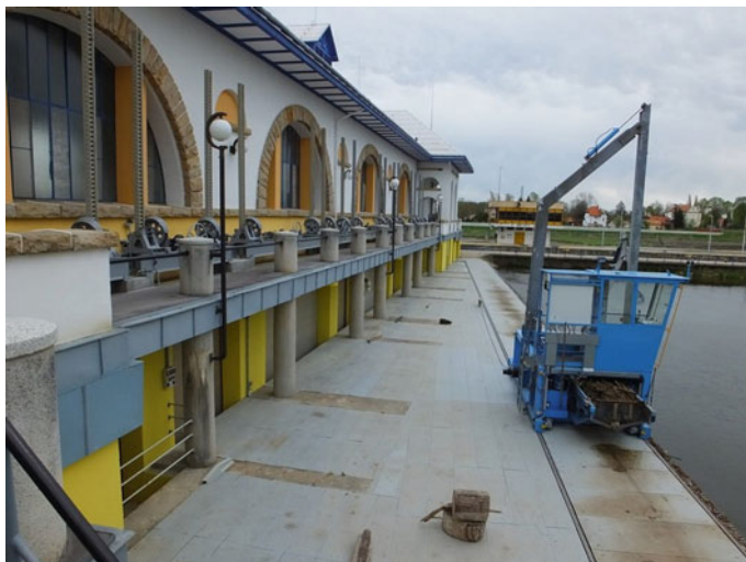
Fig. 15.14 Steel platform above the intake part of the SHPP with a new automatic cleaning machine
