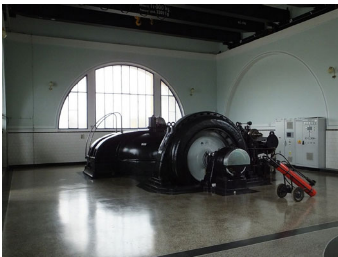
Fig. 15.15 Historical set with vertical Francis turbine in the generator hall of SHPP Mířejovice (bevel gear, generator and regulator)
