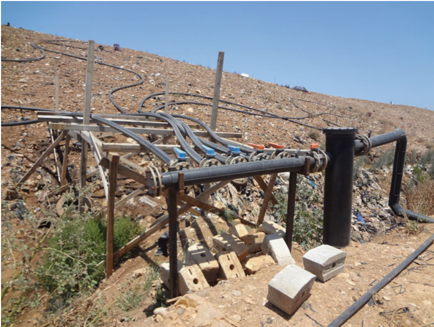
Fig. 11.6 Gas collection network in Tripoli Landfill
