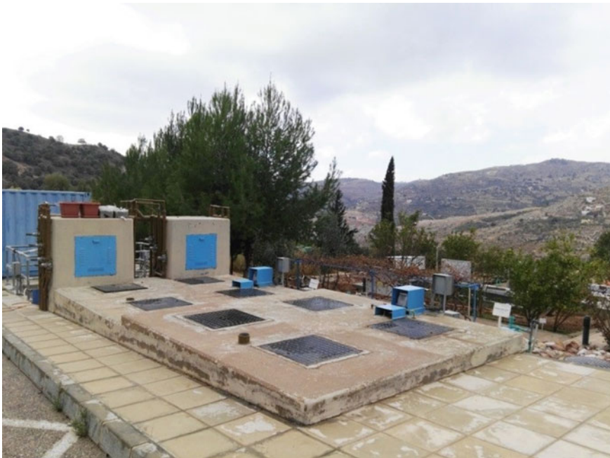
Fig. 15.6 Modified septic tanks, suspended and attached growth system at the facility site
