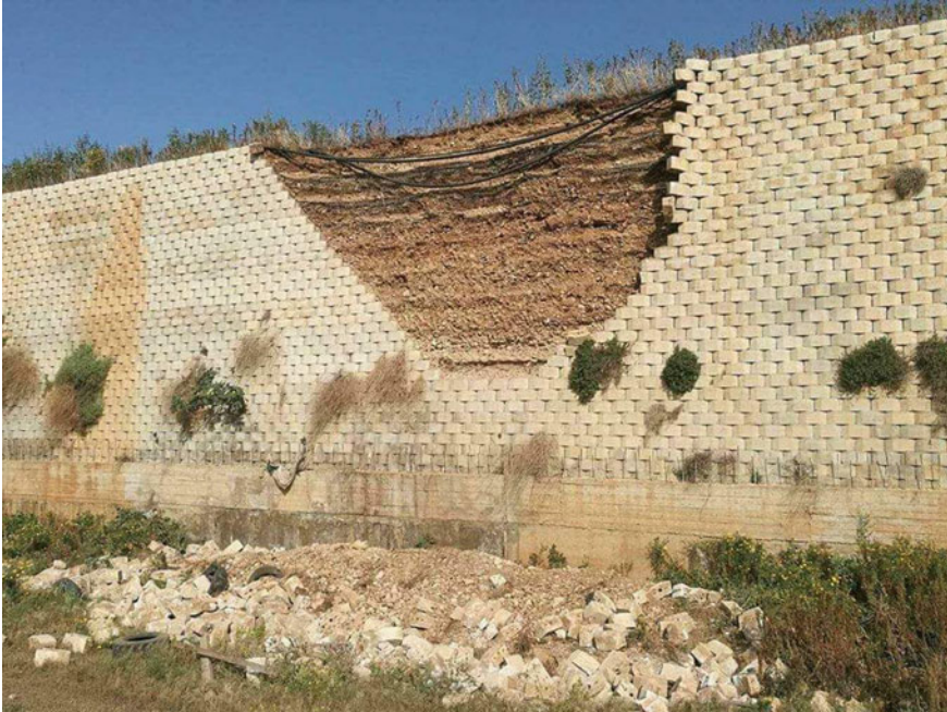
Fig. 11.8 A partial collapse in the peripheral wall
