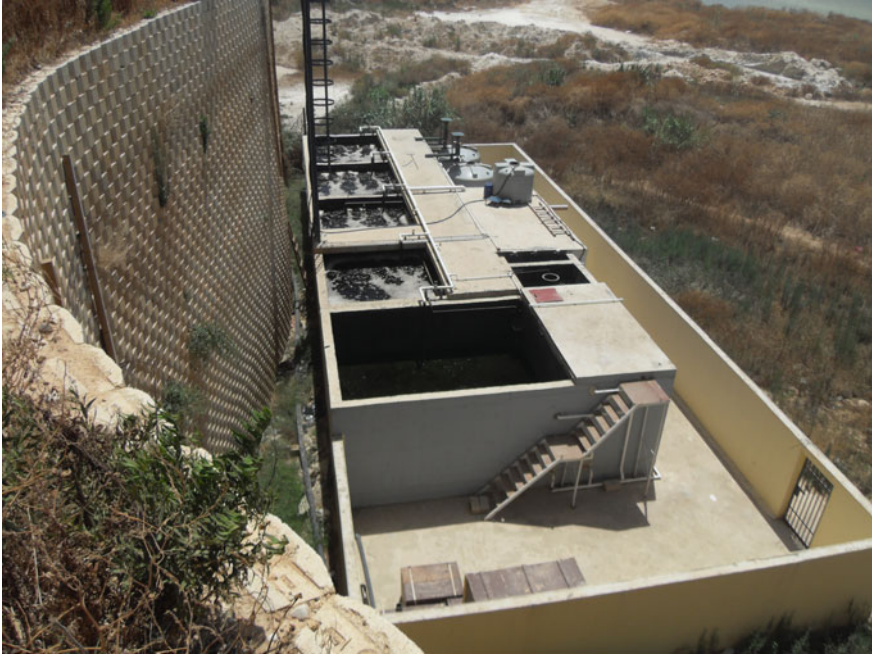
Fig. 11.4 Leachate treatment unit in Tripoli Landfill
