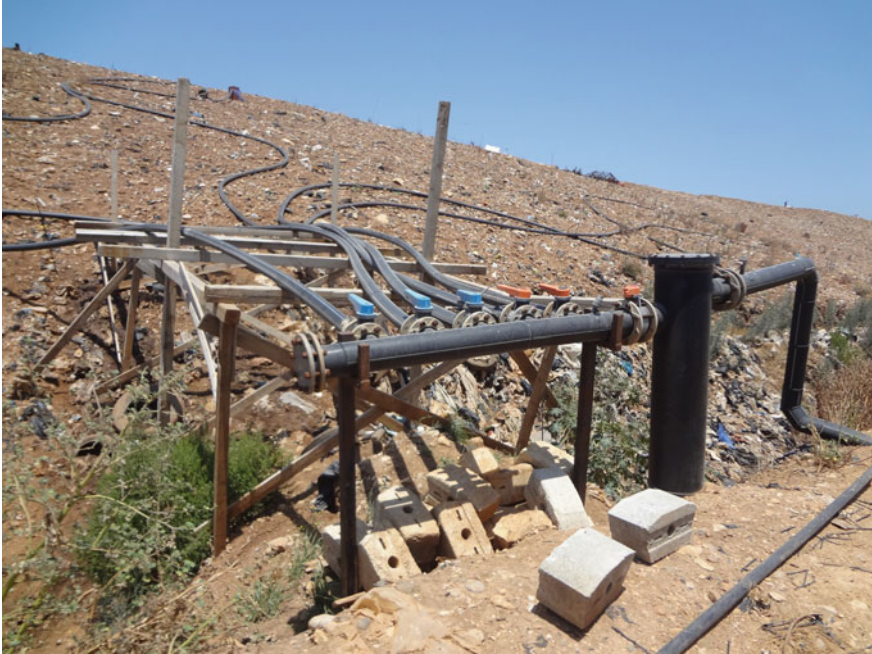
Fig. 11.6 Gas collection network in Tripoli Landfill
