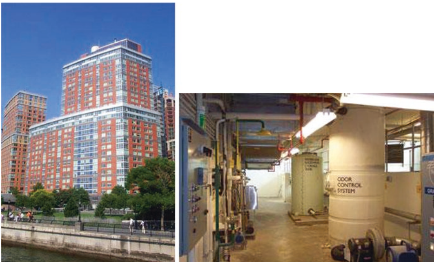
Fig. 4.2 Solaire building and on-site treatment
