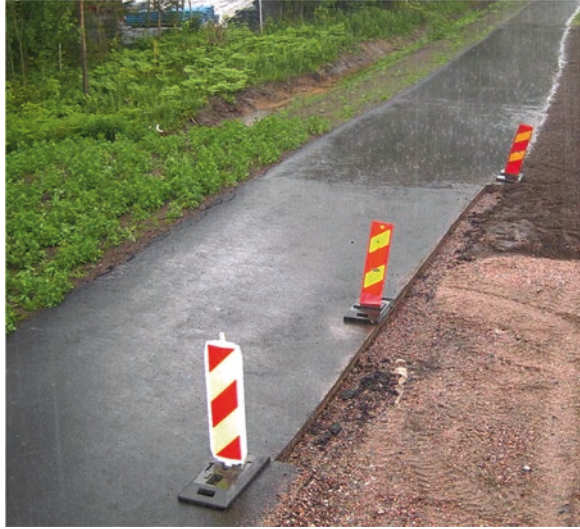
Fig. 2.4 A permeable asphalt section of pedestrian and bicycle path in Helsinki, Finland (foreground) shows reduced surface water film formation during rain events compared with conventional asphalt (background)
