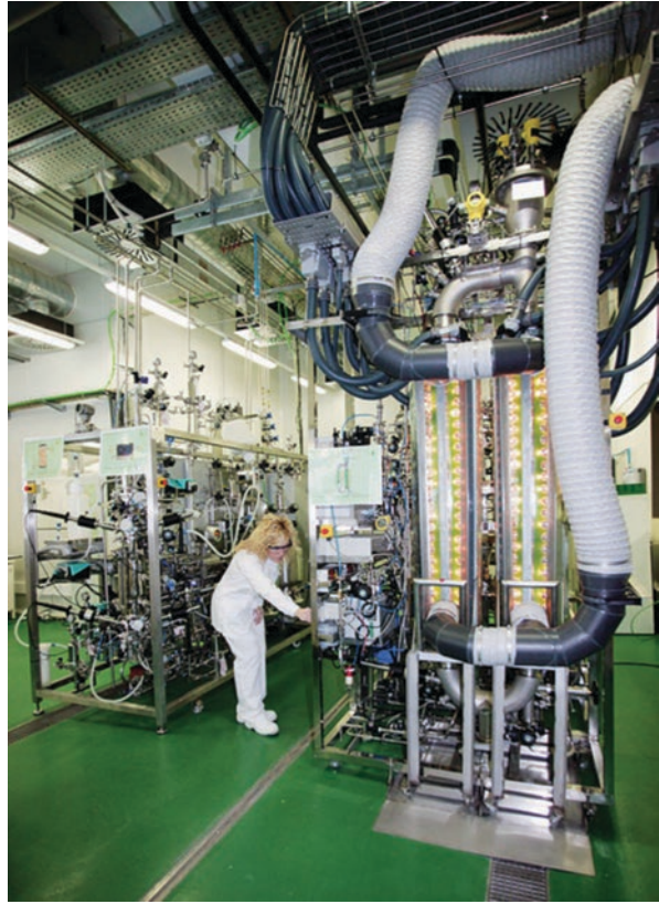
Fig. 39.4 The MELISSA pilot plant at the University Autònoma of Barcelona (image ESA)
