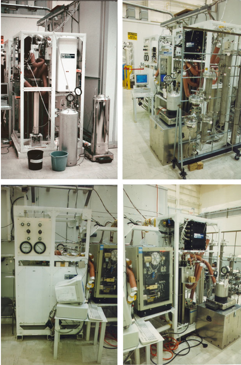
Fig. 8.41 These images show the International Space Station Water Processor. Clockwise from the upper left these images show the sequence of water processing: the stainless steel tanks which store wastewater that is to be processed and visible in the lower left quadrant of the metal rack is a particulate filter with 0.5 micron porosity; stainless steel tubes called unibeds which contain ion exchange and adsorbent resins; a catalytic oxidation reactor plus a process control monitor; and two enclosed storage tanks on the bottom half of a rack for containing the processed water. Usage of these images is courtesy of the author
