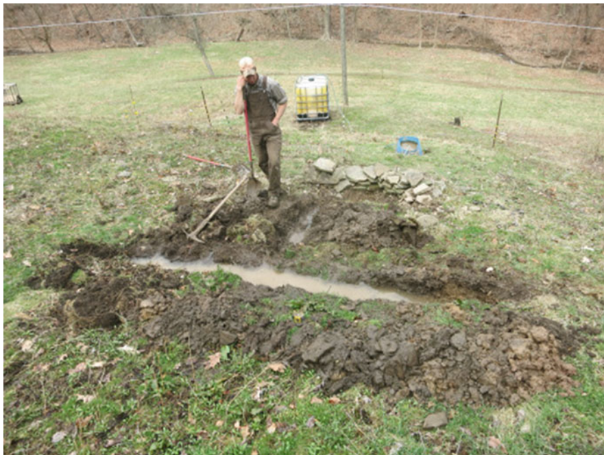
Fig. 8.8 This image shows collection of water from a seep. The water was collected using a perforated polyvinyl chloride drainage pipe. Usage of the image is courtesy of Shawn and Beth Dougherty https://onecowrevolution.wordpress.com/2018/05/13/spring-water-catching-a-seep/ . Accessed 10 Jan 2019
