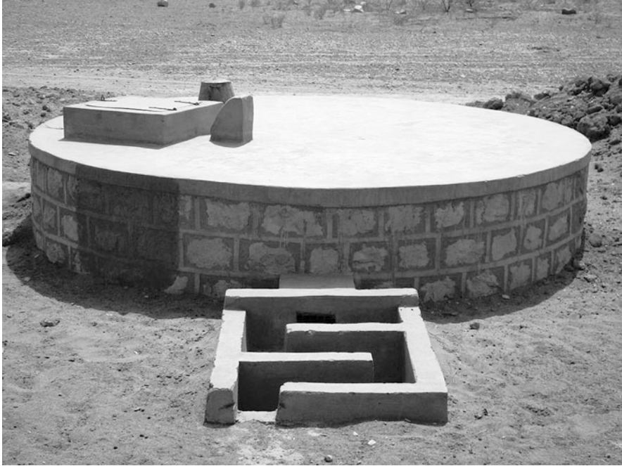
Fig. 8.10 This cistern is located in Rajasthan, India, and it is a traditional tank used for storing rainwater collected by ground catchment. The image is titled “Rainwater harvesting tank, India” by Spiritualfade and is in the public domain
