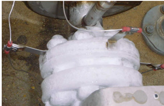
Fig. 6.18 Ice built-up on an uninsulated fitting [4]
