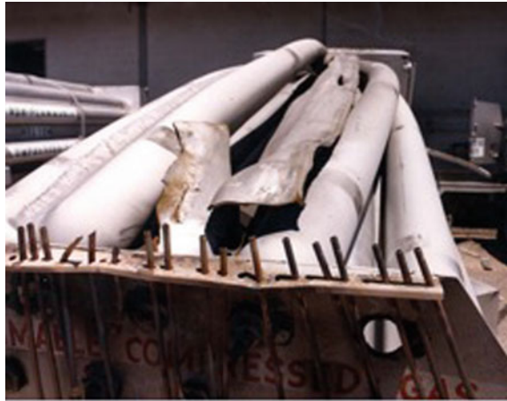
Fig. 6.1 Close up view of tube bank, post-accident [4]
