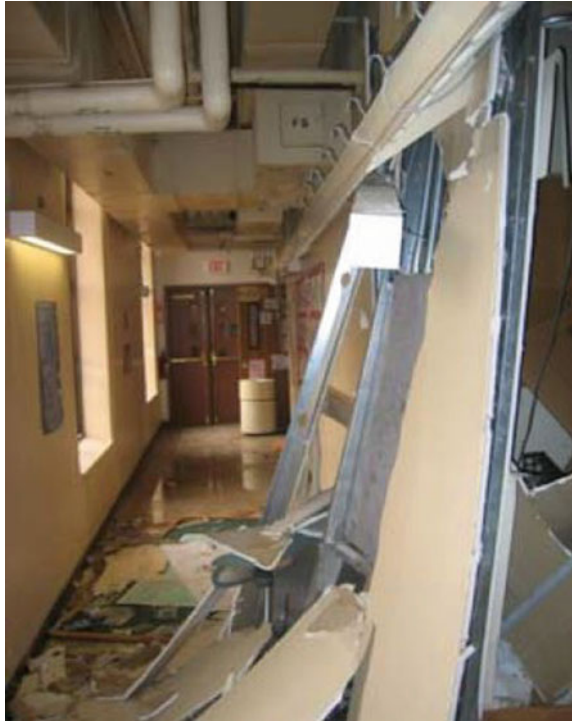
Fig. 3.2 The explosion blew the laboratory room wall out into the hallway
