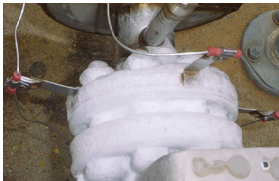
Fig. 6.18 Ice built-up on an uninsulated fitting [4]
