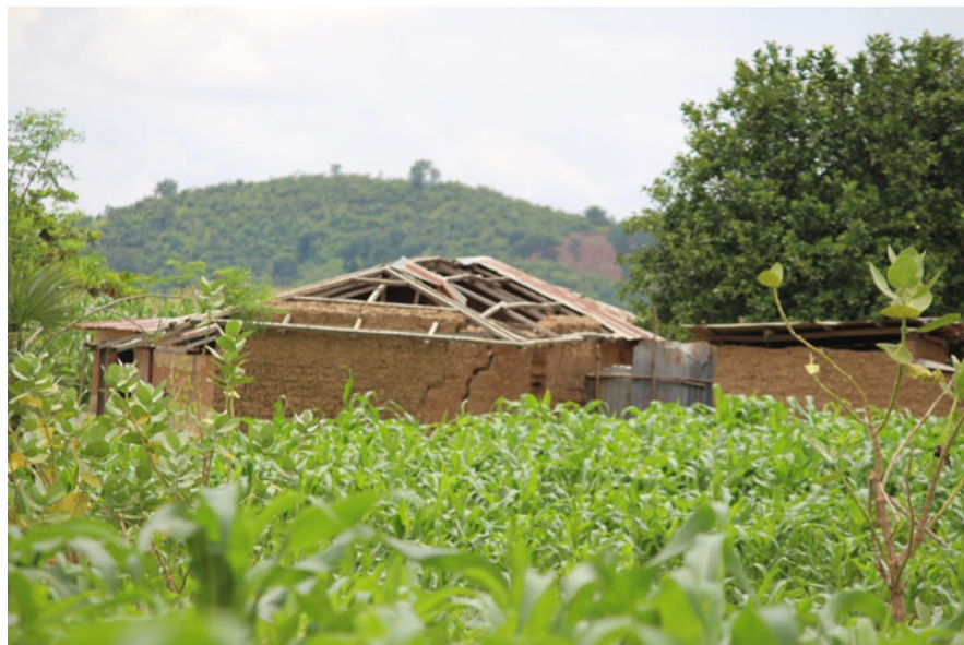
Plate 2 Image showing one of the affected houses by the 2012 flood. Source: field survey, 2013
