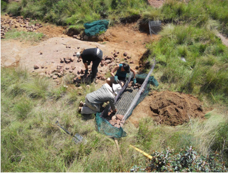
Fig. 3 NCA students packing a wire gabion basket with locally sourced rocks to slow down rain-water runoff and in the process rehabilitate a soil erosion site in Telperion Nature Reserve (© G. Wilson 2013)
