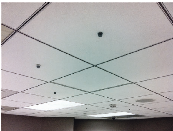
Fig. 11.1 Ceiling-mounted unidirectional and omnidirectional condenser microphones dispersed to capture all sections of the room. Note the “Voice of God” overhead PA speaker is 3 feet away from the microphones
