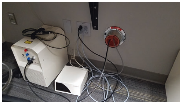
Fig. 9.1 An acoustically insulated wall conduit was installed through the wall between the simulation room and the control room to allow wires and hoses to pass. In this case, the conduit is separating the noise of the compressor used to operate the simulator from the educational environment of the room
