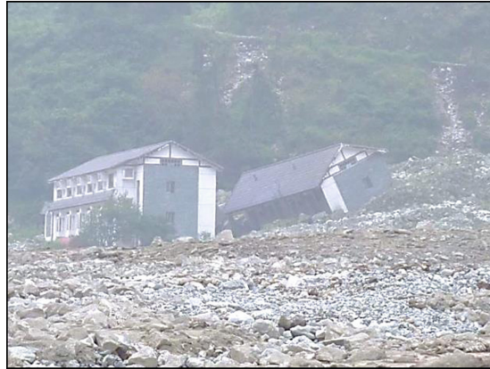
Fig. 2. Declining resistance of two buildings after subject to a strong earthquake and several debris flows.
