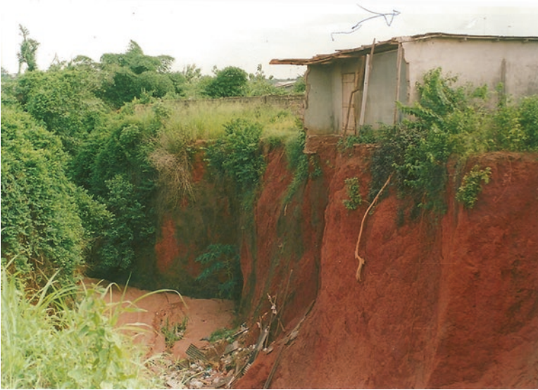
Plate 3 This building lost a large portion of it to the Odokala gully erosion
