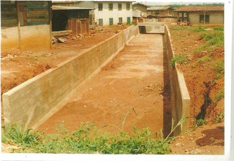
Plate 8 Channelization of the Odokala Gully: An Intervention of the Federal Government of Nigeria
