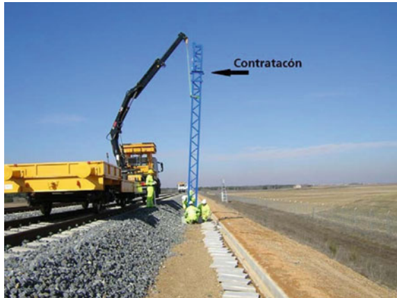
Fig. 1 Image of guided poles or vain supports
