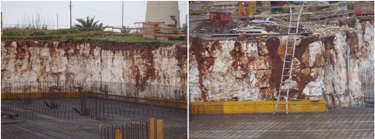
Fig. 2 Artificial cut, for construction purposes, in the Meso-Cenozoic carbonate rock mass: the epikarst portion, with many fissures and joints, tapering down and filled with residual deposits, is visible. The picture on the right shows also some ancient cavities, entirely filled with terra rossa
