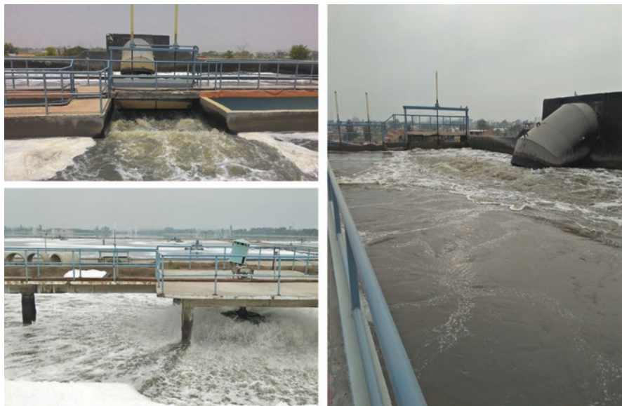
Fig. 1 Bharwarwa Sewage Treatment Plant (STP), Lucknow, India (capacity 345 MLD)
