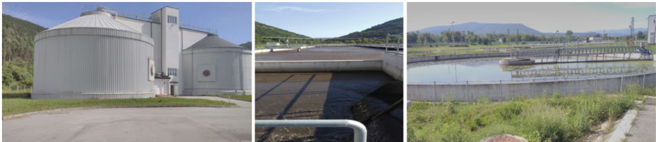
Fig. 2 Methane tanks, biobased area with aerobic and anaerobic digestion zone, secondary settler
