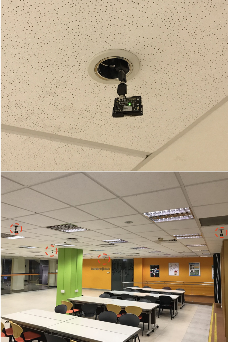
Fig. 2. Motes as deployed in the building.
