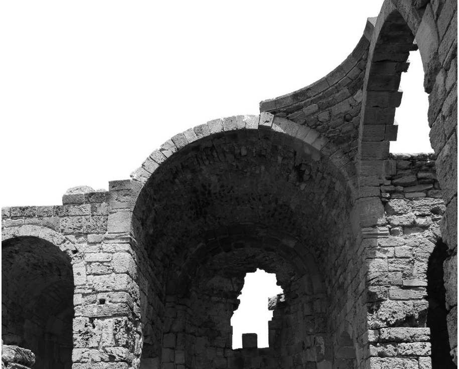
Fig. 2. Collapsed Dome in Famagusta Area, Cyprus.
