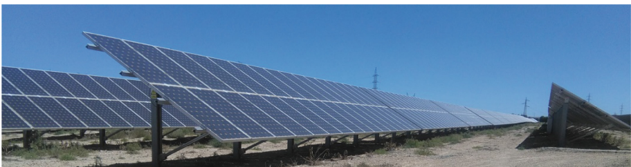
Fig. 3. General image of the 3 MW PV plant in which has been developed the research.
