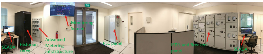
Fig. 1. EPIC control room: 360° view.
