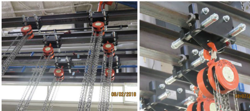
Fig. 3.16 Multi-shaker support beams, trolleys, and manual chain hoists
