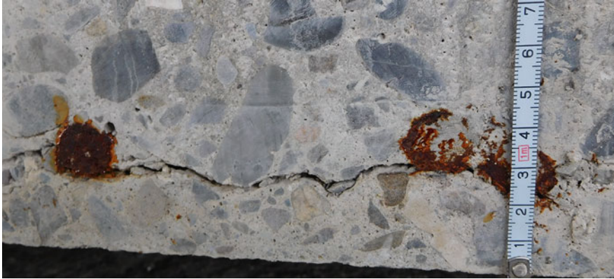
Fig. 6 Observed horizontal cracks of the cutoff deck
