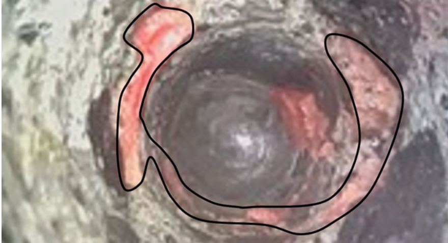
Fig. 7 Horizontal cracks observed by high-performance endoscope
