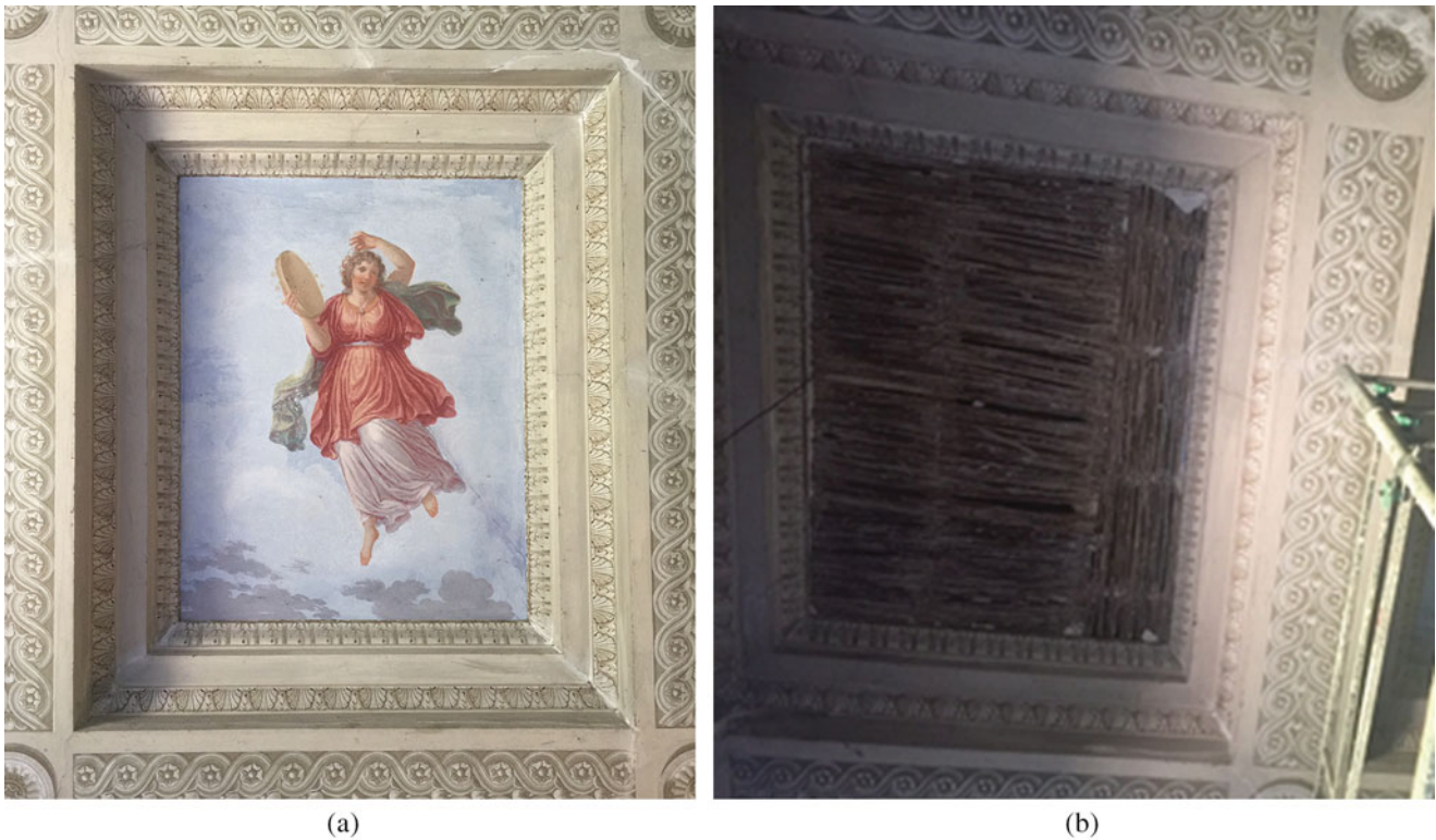
Fig. 1.3 Villa Greppi's painted loft. (a) Frescos on camorcanna. (b) Damaged camorcanna without mortar and painting
