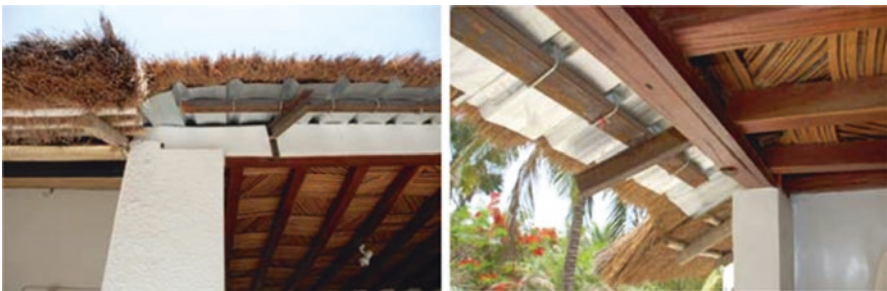
Fig. 3.55 (1 and 2) Roof with mixed construction system. The thatch is superimposed to the corrugated metal sheet (sub-layer): the benefits of sealing and durability conferred by the use of the metallic layer and the insulating ability of the thatch (tourism building, Guinea-Bissau)
