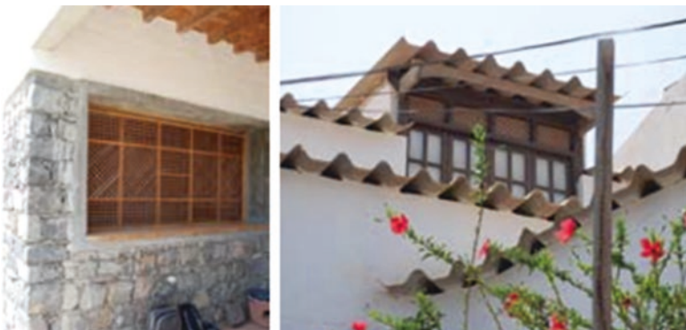
Fig. 3.72 The use of fixed grids, although not allowing adjustments to control shading and the ventilation flow, can also be an effective solution in some cases
