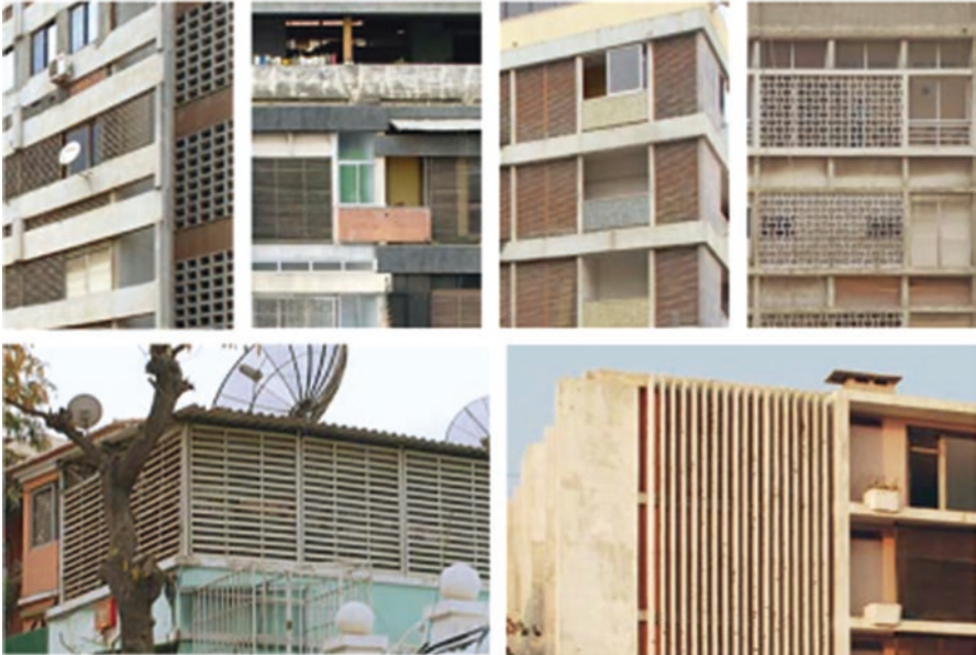
Fig. 3.66 External fixed shading systems in Luanda, Angola. As well as shading, they allow and direct the flow of natural ventilation
