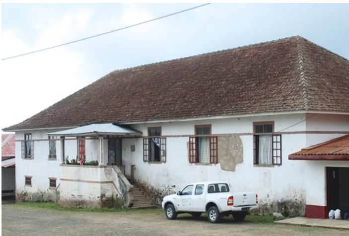
Fig. 13.10 Effects of rising dampness in a building in S. Tomé island
