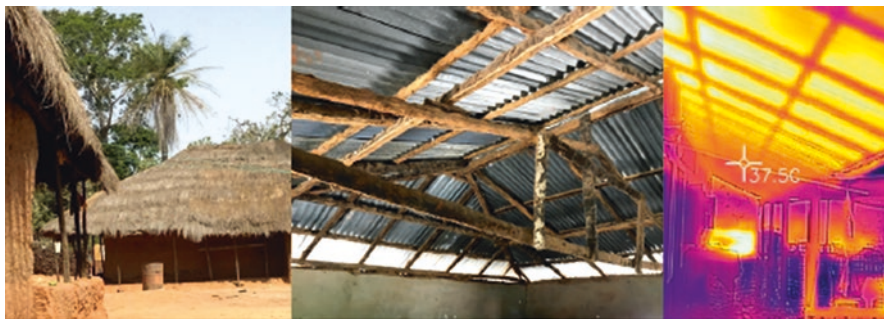
Figs. 3.131, 3.132 and 3.133 Guinea – on the left, example of a traditional roof; on the centre, example of roof with wood frame and zinc cover; on the right, thermal image of metal roof, noticing a very high heat transmission
