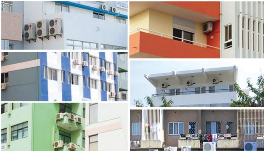
Fig. 3.148 Use of air conditioning devices, city of Praia, Cape Verde
