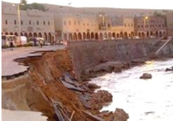
Fig. 4.15 2008 floods and destruction of the wadi banks in lower part of Ghardaia ksar
