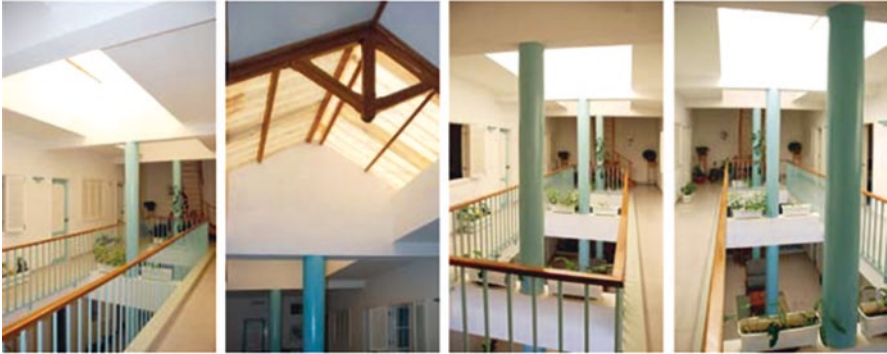
Fig. 3.87 Atrium inside a building in Praia promotes natural lighting and stack-effect ventilation. In hot climates, the top of the atrium must be at least 5 m above the occupied space and must have outlet air vents in order to prevent the accumulation of hot air
