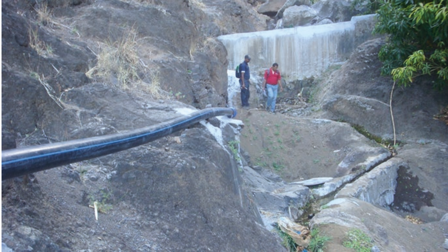
Fig. 16.2 Surface water abstraction of Figueiras, Santo Antão, Cape Verde
