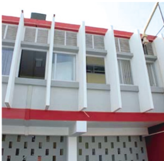
Fig. 3.73 Modernist building in Praia, with facade ventilation openings at various levels: high, for air exchange and cooling of the building mass, and lower (windows) for the comfort of occupants. The need for natural ventilation and shading was considered factors in the design of the building, which is visible in the facade typology
