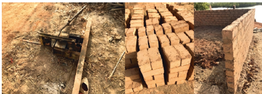
Figs. 3.122, 3.123 and 3.124 Guinea – on the left, image of a manual press; on the centre, stack of mechanical adobe blocks used for constructions; on the right, example of wall being built with this technique
