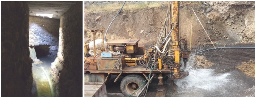
Fig. 16.3 Groundwater abstraction of São Vicente, Santo Antão (on the left) and borehole drilling (on the right) in Cape Verde
