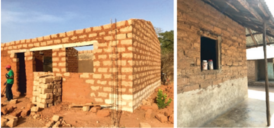
Figs. 3.136 and 3.137 Guinea – on the left, example of construction blocks with added lime to assure water resistance; on the right, application of a coating layer rich in lime, in order to protect the building foundation blocks from water damages
