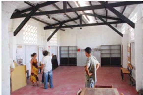
Fig. 3.86 Building for cultural activities in Lagedos. Openings at top and opposing fronts, for cross ventilation, and opening on the roof for stack-effect ventilation
