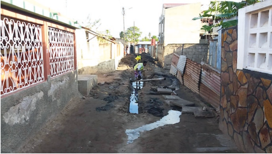
Fig. 8.8 Ongoing expansion and improvement of a gray water collector in Mafalala, Maputo, 2018. (By: Remígio Chilaúle)
