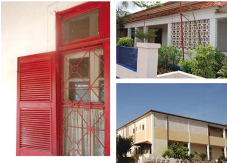
Fig. 3.67 External fixed shading systems in Guinea-Bissau. As well as shading, they allow and direct the flow of natural ventilation
