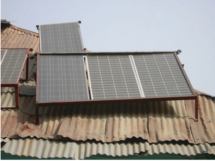
Fig. 12.2 PV individual home system in Guinea-Bissau (photo by the author)
