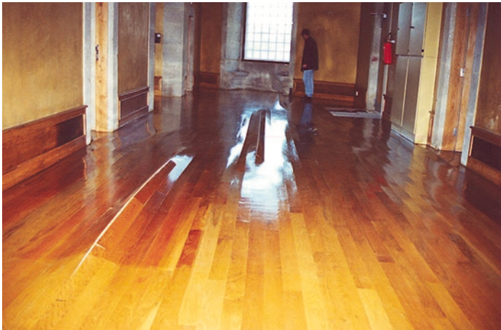
Fig. 14.3 Swelling of timber flooring after application
