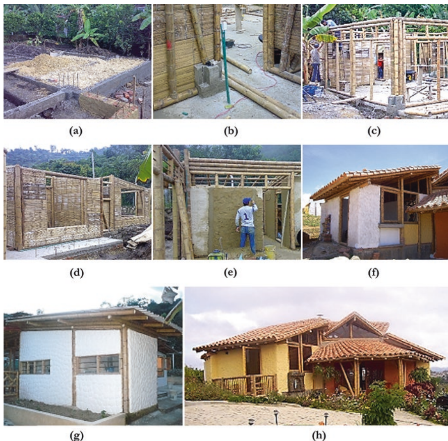
Fig. 15.8 Construction process of the plastered cane wall framing system (picture (h) by Arme Ideas en Bamboo Ltd). (a) Foundations. (b) Anchorage. (c) Framing and bracing. (d) Sheathing with riven bamboo. (e) Rendering. (f) Roofing. (g) Finishing. (h) Final product
