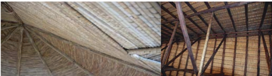
Fig. 3.57 Internal roof insulation in a recent building, using local materials (thatch), in Guinea-Bissau (left) and Mozambique (right)
