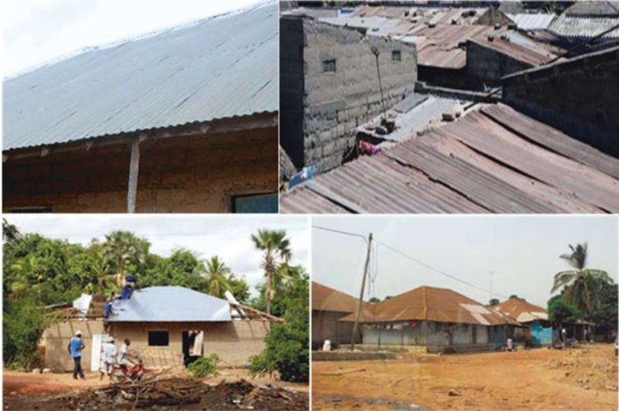
Fig. 3.56 Guinea-Bissau: The use without protection (insulation) of metal roofing should be avoided since it leads to situations of internal overheating. Furthermore, with the oxidation, the metal cover darkens, transmitting more heat to the internal spaces
