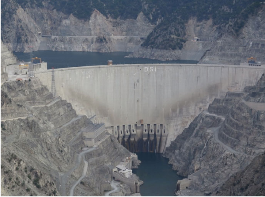
Fig. 12.8 The 249 m high (above foundation) Deriner dam on Chorokhi (Coruh) river. (Photo by Y. Ozdemir)
