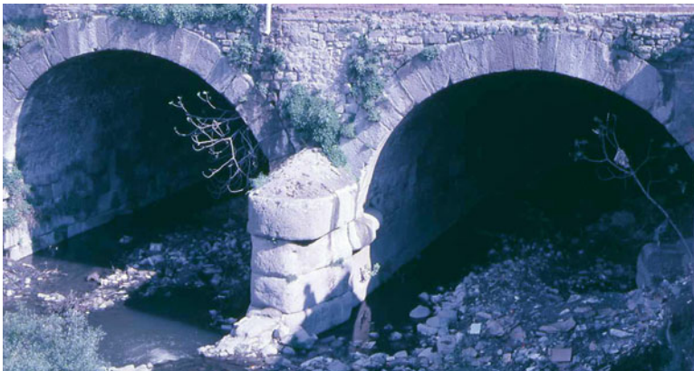
Fig. 2.23 Inlet of the twin structures covering the Bergama Creek. (Photo by U.Ozis)
