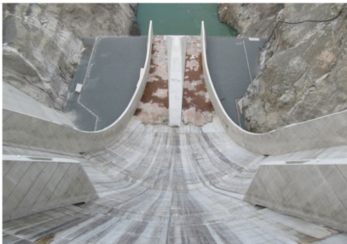
Fig. 12.9 The 190 m high (above foundation) Artvin dam on Chorokhi (Coruh) river. (Photo by Y. Ozdemir)
