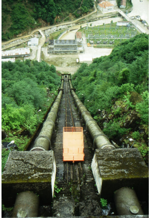
Fig. 10.6 Dogankent-A power plant, penstocks of 1.85 m diameter, on Harsit river. (Photo by U. Ozis)
