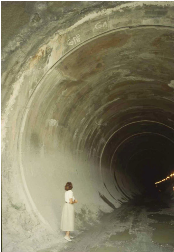
Fig. 12.20 The Sanliurfa twin tunnel, fed from the Ataturk dam’s reservoir. (Photo by U. Ozis)
