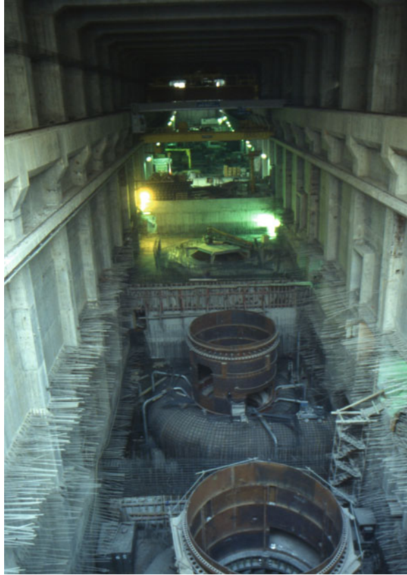
Fig. 10.3 Ataturk power plant of 2400 MW during construction of eight units at various phases. (Photo by U. Ozis)
