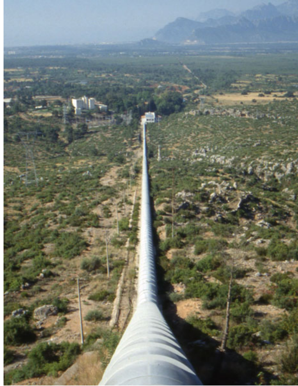
Fig. 10.14 Kepez I high-head diversion scheme and penstock in the direction of Antalya Bay. (Photo by U. Ozis)
