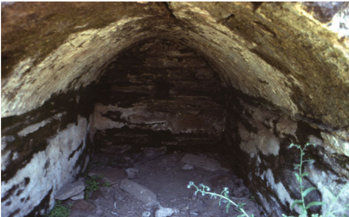
Fig. 2.13 A springwater collection chamber of the water conveyance to Alabanda. (Photo by U. Ozis)
