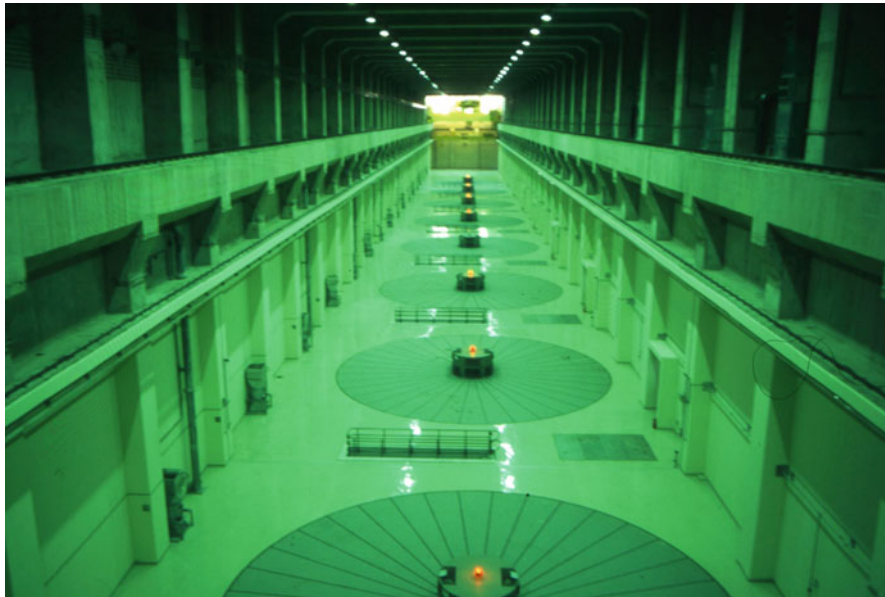
Fig. 10.15 Ataturk indoor type powerhouse. (Photo by U. Ozis)
