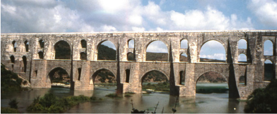
Fig. 2.28 Maglova Aqueduct-bridge on the Kirkcesme Water Conveyance to Istanbul. (Photo by U.Ozis)
