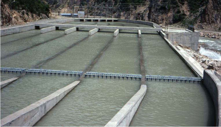
Fig. 10.11 The desilting basin of the Dogankent high-head diversion scheme on Harsit (Photo by U. Ozis)
