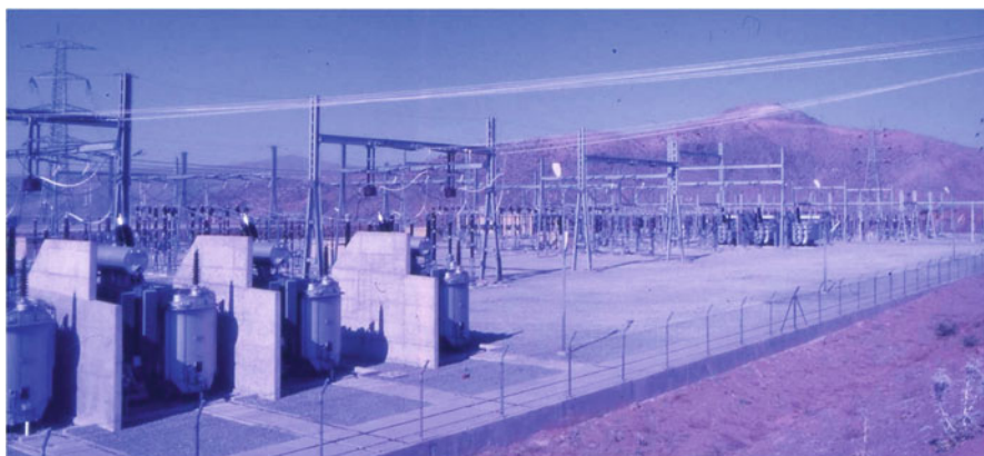
Fig. 10.23 The main switchyard of the Karakaya hydroelectric power plant, which is the link to the interconnected transmission network of Turkey. (Photo by U. Ozis)
