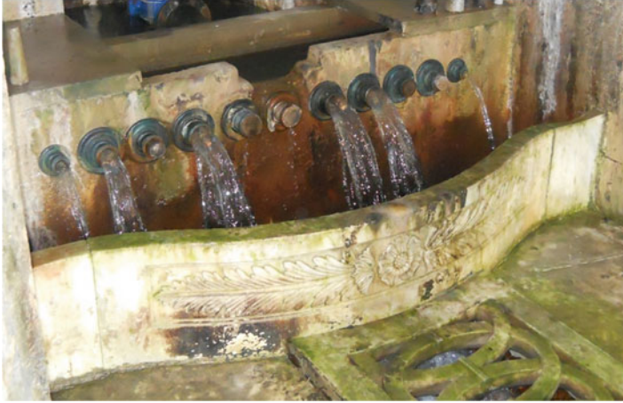
Fig. 2.26 The Orifices (lule) in the operation chamber of the Yeni Dam. (Photo by Y.Ozdemir)
