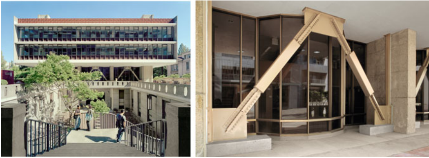
Fig. 2.6 Prior to seismic retrofit the structural system of the Hildebrand Hall lacked shear-resisting elements. The architects Anshen and Allen and structural engineers Forell/Elsesser decided for the strategy of seismic strengthening through the use of unbounded braces made of steel and concrete in combination with additional shear walls [14] (photographs by Forell/Elsesser)
