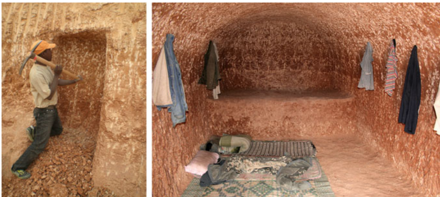
Fig. 5 The construction of a single room in Kabaw, Libya (Picture by B. Polimeni 2011)
