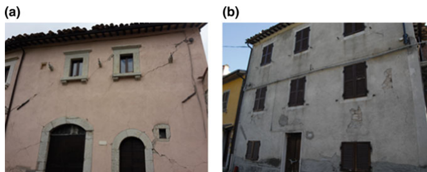
Fig. 3 Favorable behavior of masonry structures under seismic actions. In-plane damage limited to repairable elements without collapse (mode 2): shear failure mainly extensive in masonry piers a (Castelsantangelo sul Nera) and, more favorably, on lintels b (Pieve Torina, MC)
