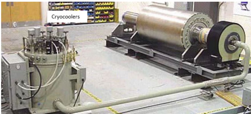
Fig. 6.27 Separate cold box with transfer line to generator by AMSC [35]
