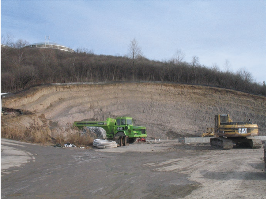
Fig. 15.4 Extensive site modification is possible by using heavy machinery. Here part of a hillside and associated vegetation was removed to make room for a new building. The slope was ultimately stabilized with a large retaining wall complex. (Source: Tim Toland)
