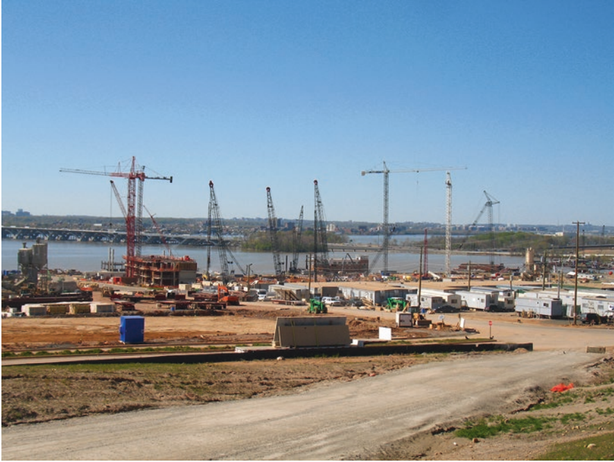
Fig. 15.1 Site development: site project along a river that involves a significant number of earthwork and construction activities by heavy equipment. The site underwent extensive shaping to get it to fit the final design. Extensive environmental protections would be required in a project such as this. (Source: Tim Toland)
