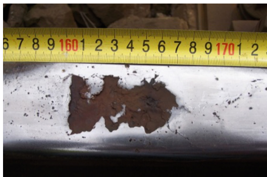
Fig. 3. Measurement of defects.
