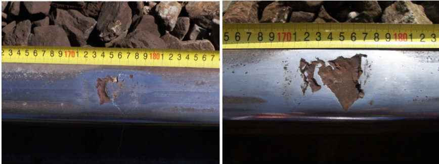
Fig. 4. Development of defect in the rail over a period of 15 months of rail exploitation.
