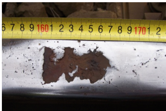
Fig. 3. Measurement of defects.
