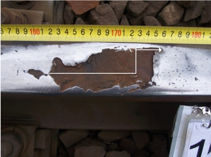
Fig. 7. Defect with a significant length and a significant width.
