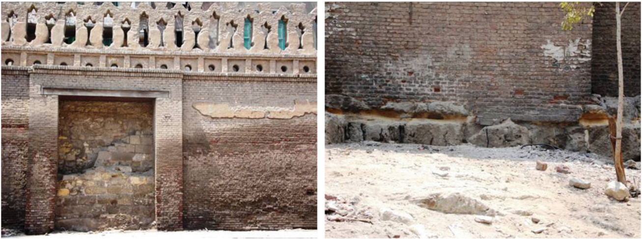
Fig. 4 Decay on the walls and fences of the mosque
