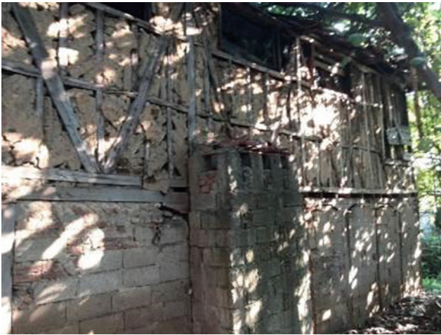
Fig. 51 Improper materials on the walls
