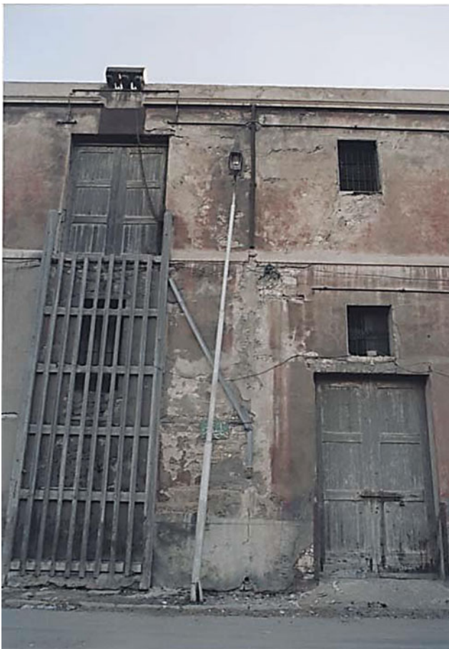
Fig. 11 Ruined warehouses. Photograph at present taken by the author
