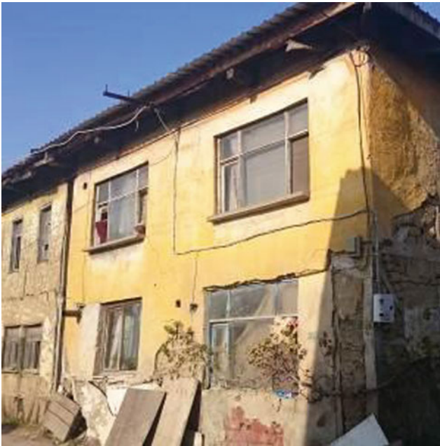
Fig. 52 Inappropriate changes of windows
