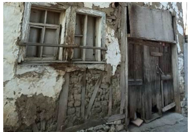
Fig. 50 Loss of fillings and plasters
