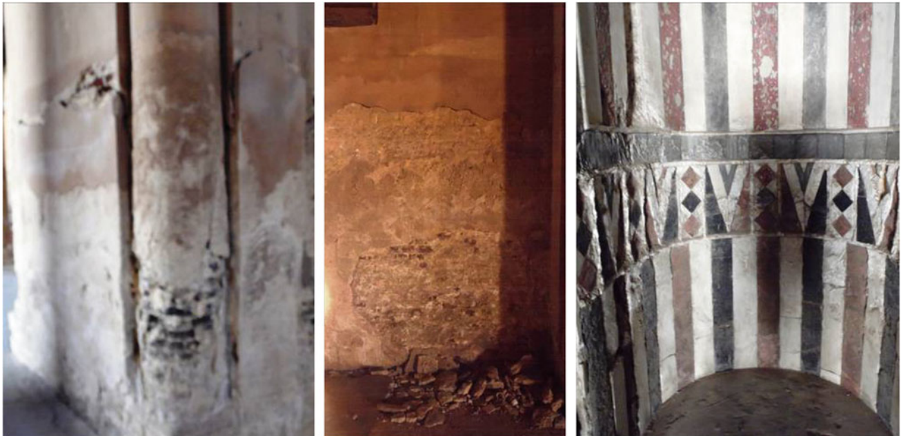
Fig. 5 Some decay and cracks on the walls and bovines of the mosque
