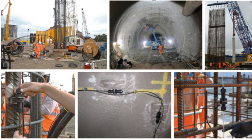
Fig. 14 Installation of optical fiber cables for monitoring distributed strains in pile, tunnel and diaphragm wall
