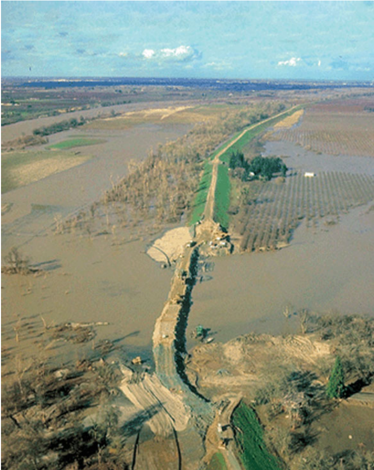
Fig. 9 A broken levee under repair in the Sacramento River delta (from [39]). California has more than 21,000 km of levees to protect dryland from floods
