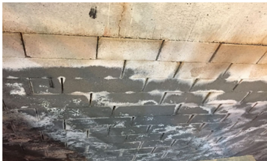
Fig. 15 Refractory condition after 12 rounds of fire
