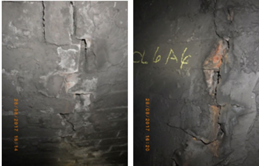
Fig. 5 Cracking behaviour of first design tested
