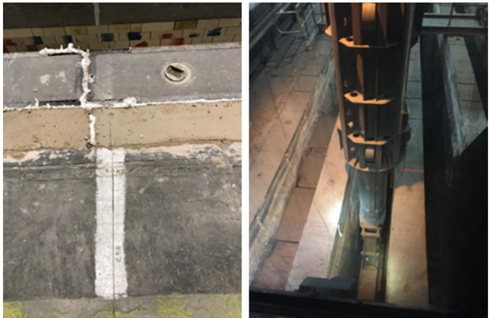
Fig. 13 Marking on the tub wall (left) and laser line shown on flue top (right) to assist with anode packing
